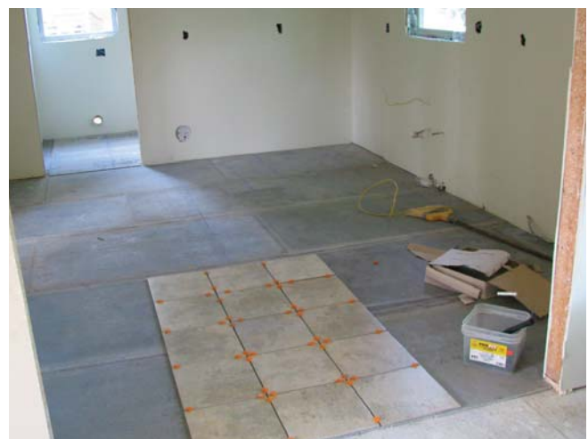
(Fig.20) Tile can be installed by professionals or homeowners. Shown here, 12" ceramic tile is being installed by skilled and unskilled volunteers.
