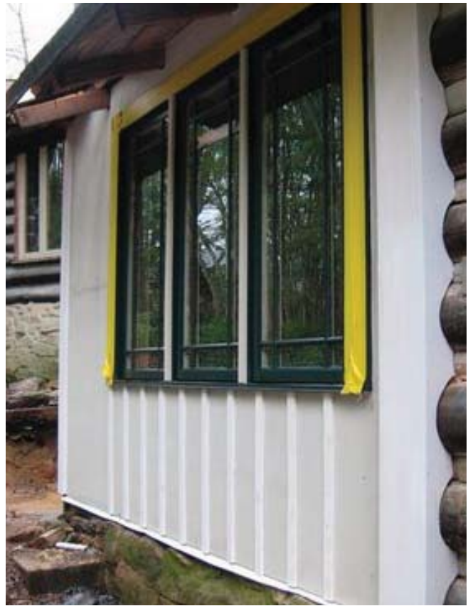
(Fig.6) Fiber-cement vertical panels are used above in a cabin addition. 1x battens are used on the vertical joints between panels. Many fiber-cement products are primed at the factory.
