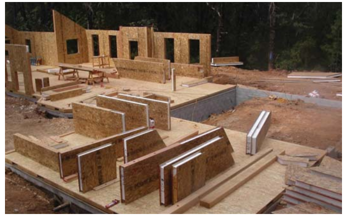
(FIG.A) PANELIZED SYSTEMS are delivered to the site as a package. Builders familiar with SIP construction can erect the structure quickly, reducing labor costs.
