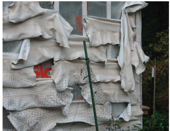
(Fig.9) Vinyl siding has a very low melting point. Here, a house fire caused the vinyl siding to melt, releasing toxic fumes.
