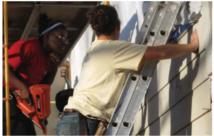
(FIG.A) EXTERIOR FINISHES of walls should be well-secured in order to withstand a high wind load. Here, fiber-cement siding is nailed through the sheathing to the framing members, over a vapor barrier.
