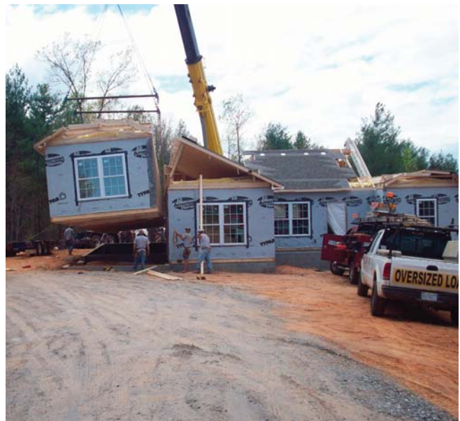
(Fig.3) The weight of modular units requires that they be lifted into place with a crane. Professional crane operators and modular installers must be used to ensure safety.
