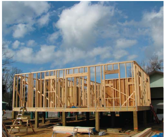
(Fig. 2) With an experienced crew, a house can be framed in a matter of days.
