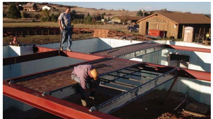
(FIG.C) SUSPENDED CAST-IN-PLACE DECKS can be used in combination with ICF walls and a concrete foundation system.
