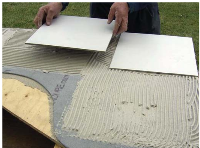
(Fig. 35) Ceramic tiles are set in a layer of mortar. In this case, magnesium oxide panels are used as the tile backer board.
