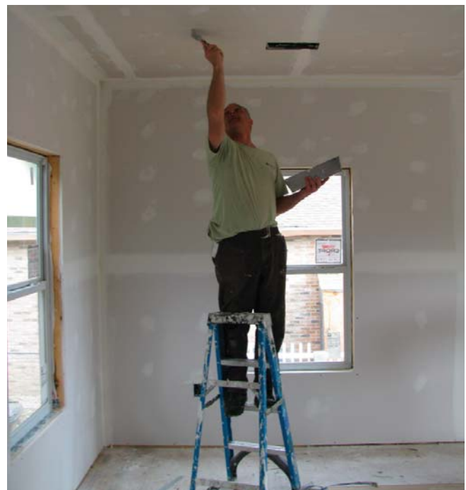
(Fig. 24) Gypsum board finishing (taping and floating) is the process in which panel joints, screw and nail holes, and other imperfections are concealed to create a smooth surface.
