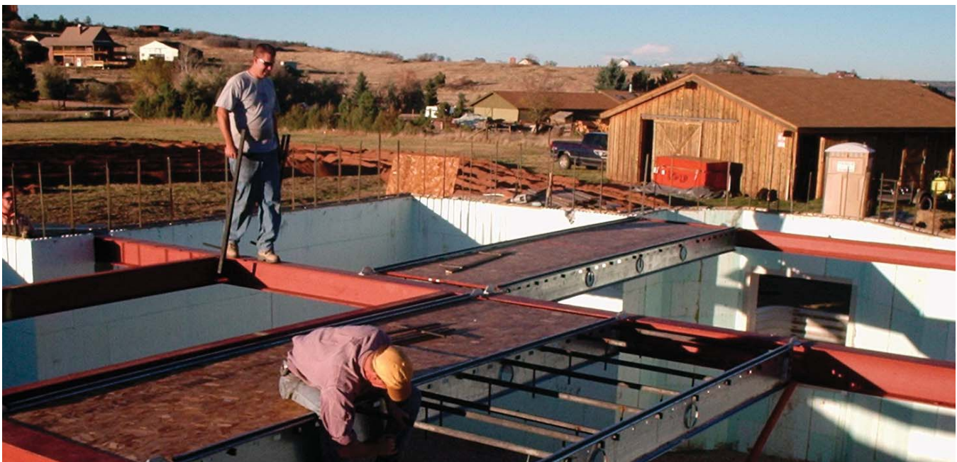
(Fig.4) Reusable steel lockbars being set into the joists. These lockbars support the plywood while the concrete is being poured and are removed after installation.
