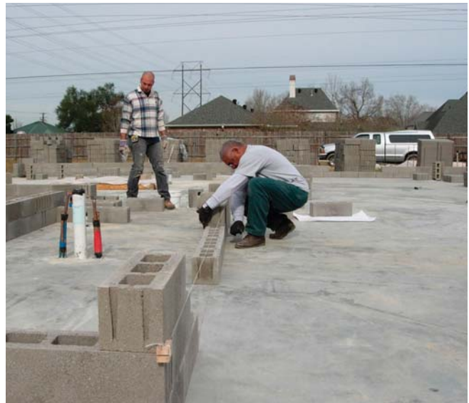
(Fig. 8) A stringline is used to lay the first course of a CMU wall.
