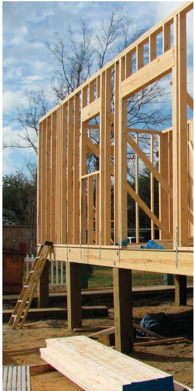
(Fig. 1) A wall and doorway are shown framed in at a house on Mississippi's Gulf Coast
