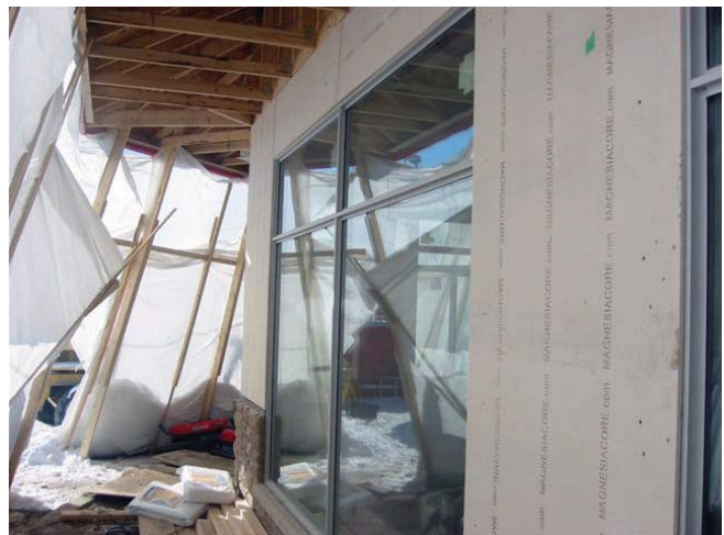
(Fig. 29) Magnesium oxide panels are used as the exterior sheathing in this restaurant.
