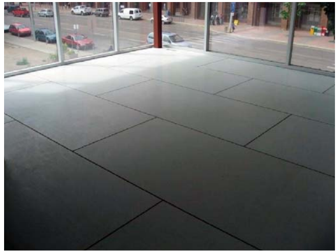
(Fig. 27) Magnesium oxide panels are used as the subfloor in this building.
