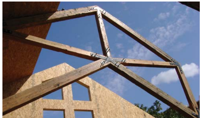
(Figs. 10-13) Process photos from Florida State University Energy & Sustainability Center's "Off-Grid Zero Emissions Building."
