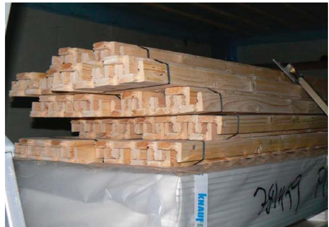
(Fig. 11) Finger jointed i-beam engineered studs arriving on-site in a lumber package delivery.
