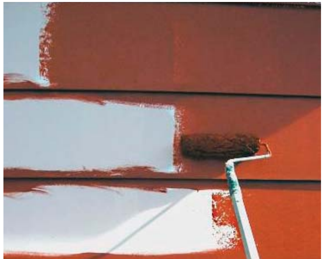
(Fig.1) Masonite siding should be painted every few years to protect from water damage, mold, and rot. Special attention should be paid to the bottom edge of the exterior lap, where damage often occurs.
