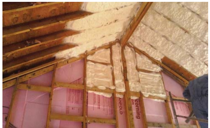
(FIG.C) INSULATION helps maintain the temperature of the conditioned area within a building. This photo shows spray foam insulation sprayed onto existing rigid foam insulation to increase the R-value of the wall.
