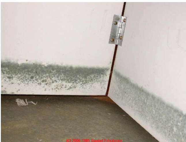
(Fig. 25) Gypsum Board with mold growth caused by flooding.
