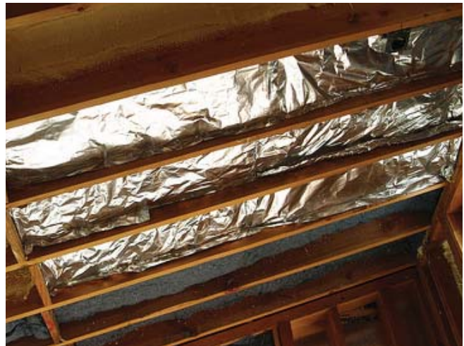
(Fig.6) Radiant barriers are often installed between roof rafters. This is an example of a radiant barrier type that could be installed in an existing building.
