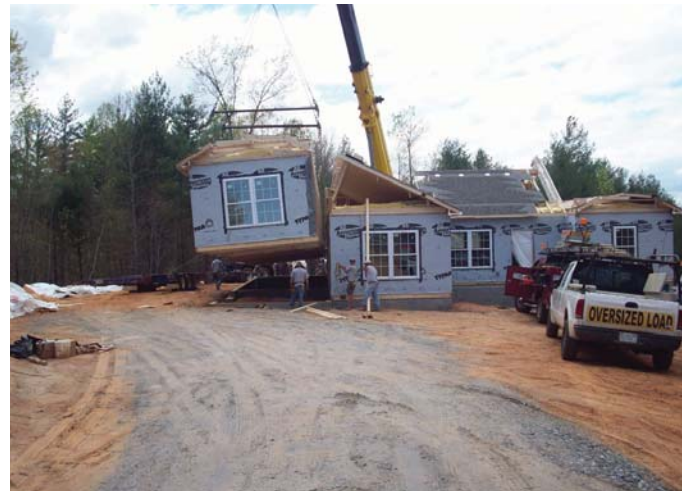
(FIG.A) MODULAR HOMES can be made of one, two, or more modules. Each module is typically completed in a factory, set in place, and finished on-site.
