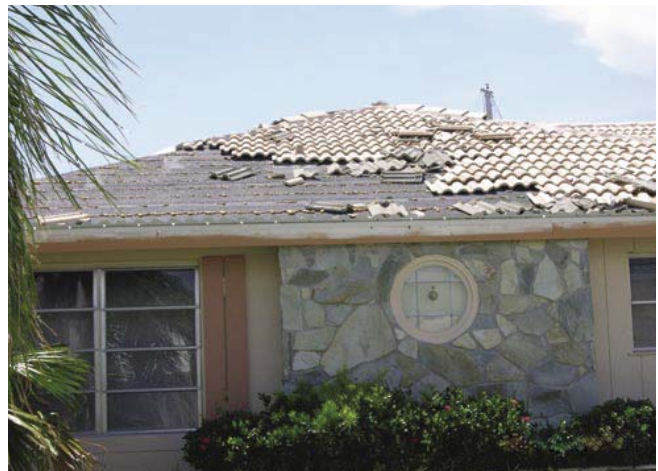
(Fig.19) Tiles ripped from a roof in a storm can become projectiles likely to damage other area of the roof. They can also cause damage to persons and structures.
