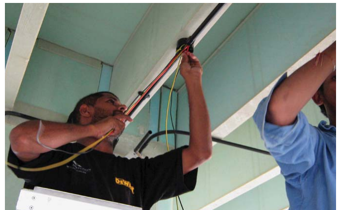
(FIG.C) INSTALLING electrical, mechanical, plumbing, or other systems may require planning ahead. Coordinate with tradespeople to avoid delays or cost overruns.
