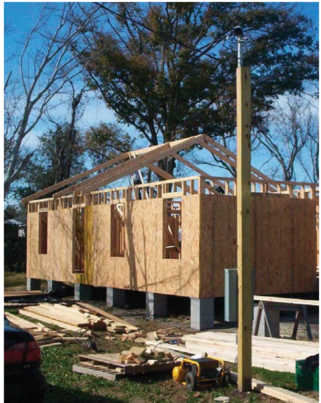
(Fig. 12) Aside from basic carpentry knowledge, no specialized labor is needed for sheathing a house.
