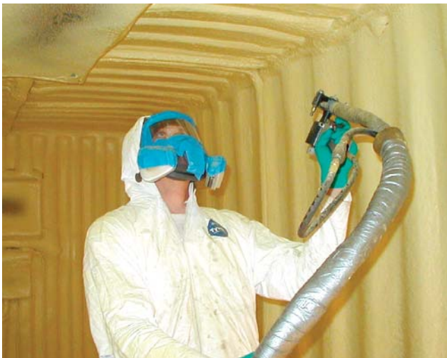
(Fig. 19) Above, open-cell spray foam insulation is installed by a professional. The excess foam will be trimmed and discarded.
