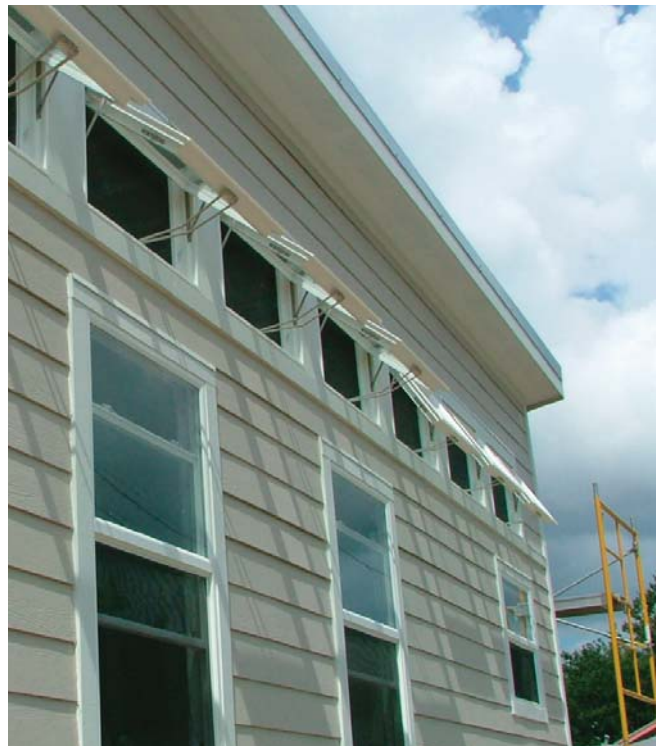
(Fig.7) Fiber-cement lap siding has the finished look of wood siding. Here, it is used in combination with fiber-cement window trim.
