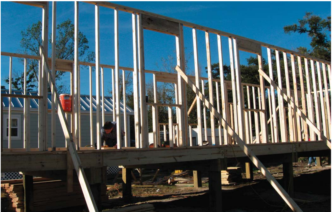
(Fig. 5) Exterior walls are held plumb by bracing until interior walls are framed.
